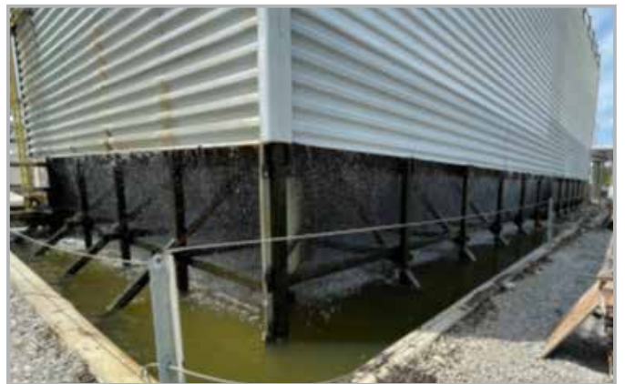
Back corner of the cooling tower basin two months into the trial. The water fall and wind circulation improved after SurfClean 2.0 application, indicating cleaning of the cooling tower fill.
