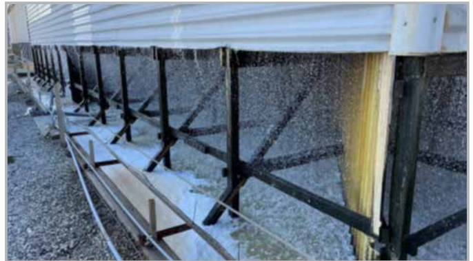
Back corner of the cooling tower basin before the trial.
