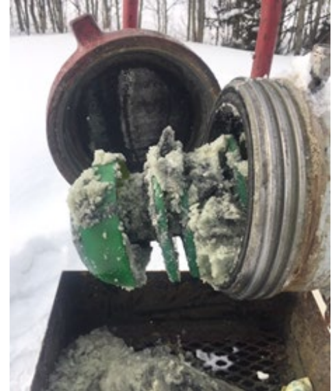
Figure 3: Pig receiver during third week with continuous treatment.
