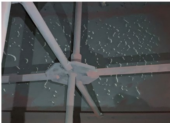
Tiger stripe pattern indicating two-phase flow-accelerated corrosion prior to FFA treatment
