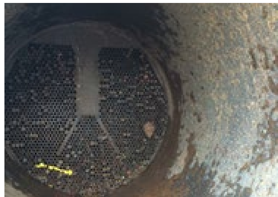
One year after FlexPro® treatment began
