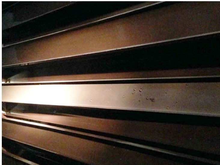
Figure 2: Deaerator trays with non-wetted surface and beaded water droplets.
