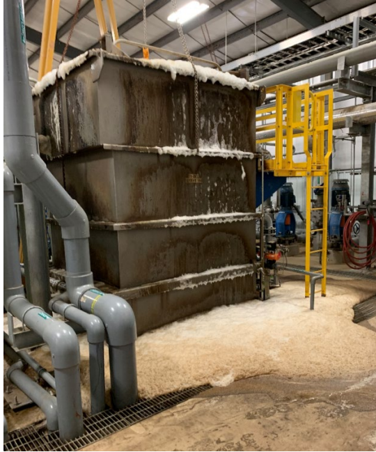
BEFORE: Excessive foaming at the pretreatment plant
