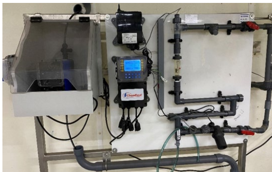
Control panel with associated equipment
