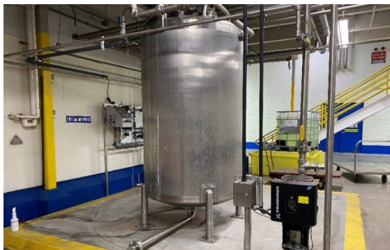
Overview of system, including control panel, mixing tank, and chemical tote
