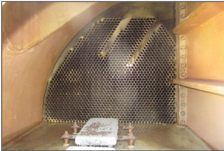
New Process Unit Heat Exchanger Cooling Water Side with FlexPro® Treatment
