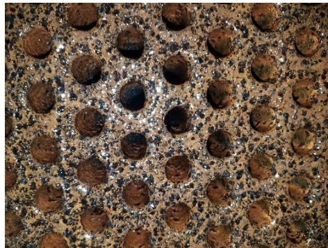
Figure 1: Photo of tube sheet after cleaning and before treatment optimization. The photo shows the extent of the previous damage and signs of additional corrosion resulting from inadequate anodic protection.
