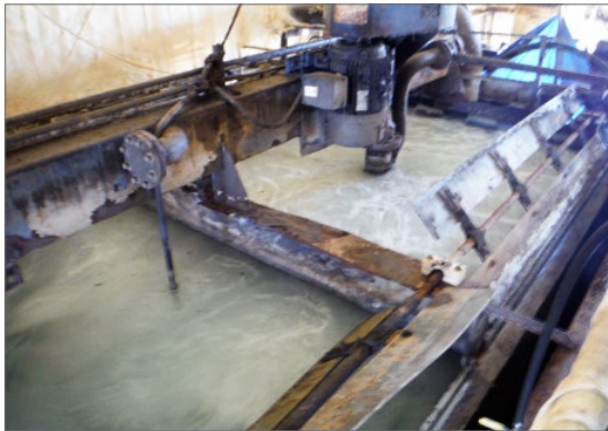
Old IAF – Induced Air Flotation Unit
