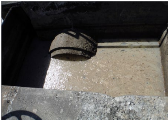
Oil Spill Event: Cast House Sluice
