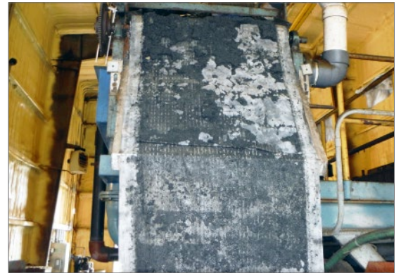
Old Hoffman Filter for Sludge Drying Off IAF
